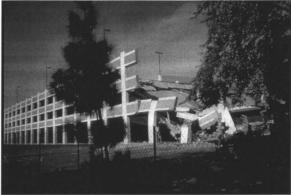
Figure 2.5 Collapse of center columns, floors and external moment frame of a parking structure at Northridge [2].
