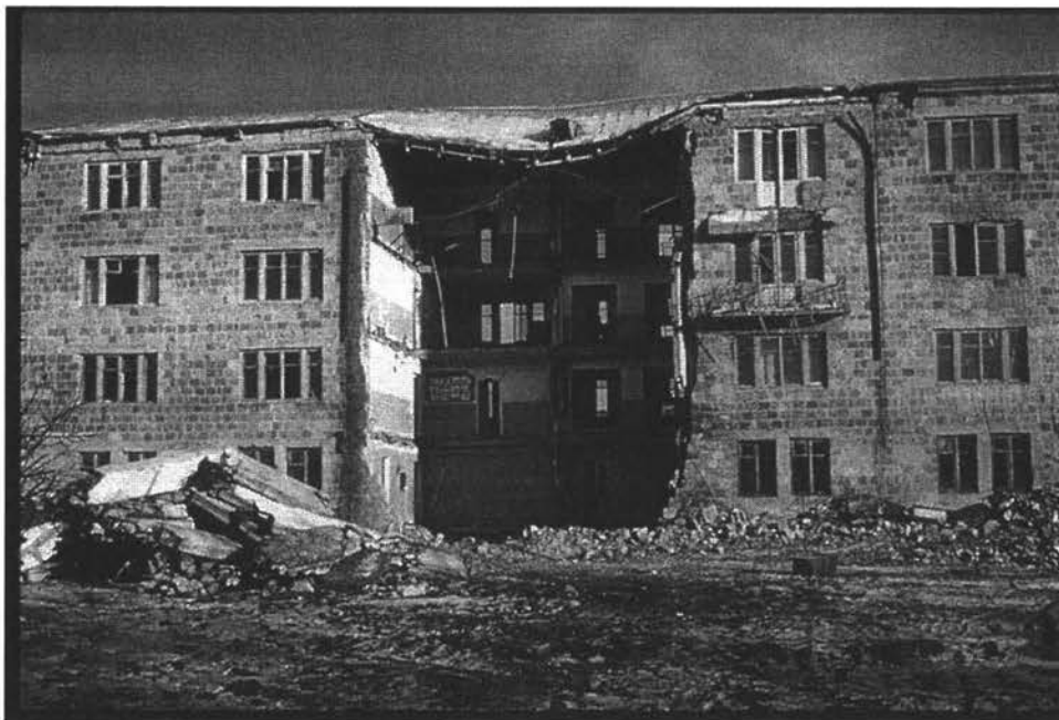
Figure 2.3 Damage to a four-story building in Leninakan due to inadequate connection between precast floors and walls [12].
