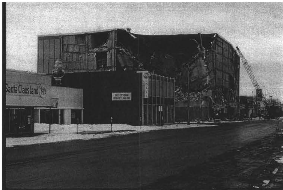
Figure 2.1 Partially collapsed building with poorly connected precast floor panels [12].
