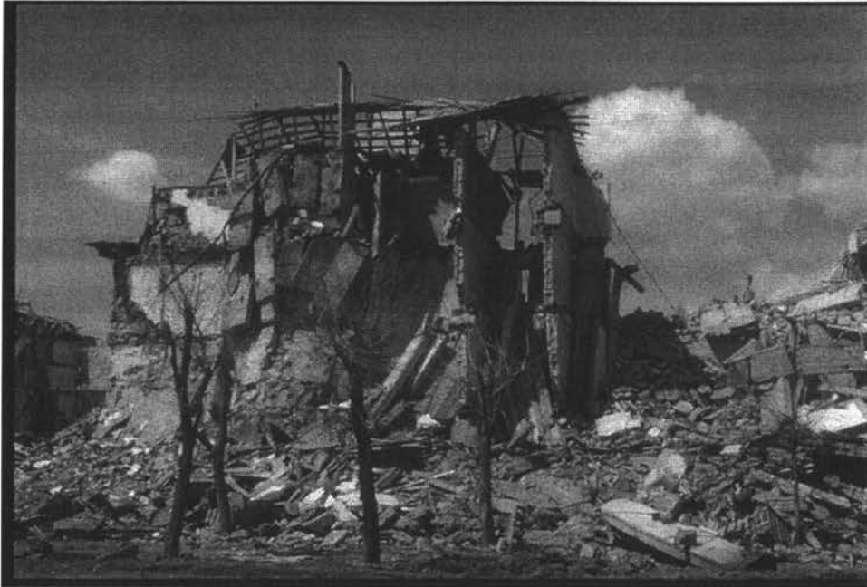
Figure 2.2 Collapse of floor panels, leaving cast-in-place walls standing in a building in Leninakan [12].
